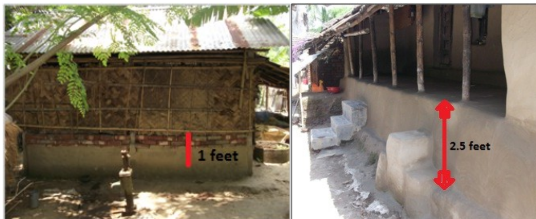
Figure 6. Raised plinth after 2012 waterlogging
